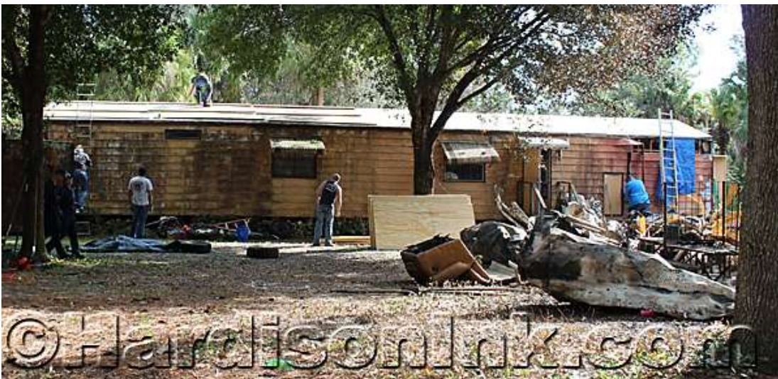
The neighboring singlewide mobile home suffered damage, but with the restoration and repair work by a strong set of volunteers, this home was saved for the Taylor family.
